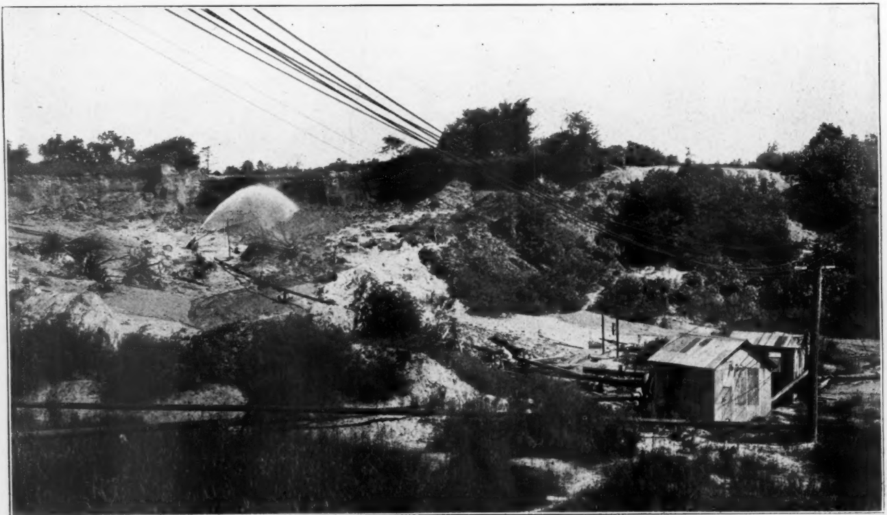
Upper Left Shows Motor Truck Loading Under Steel Bins. Lower Shows Pump House and Jet Operating Against Bank
